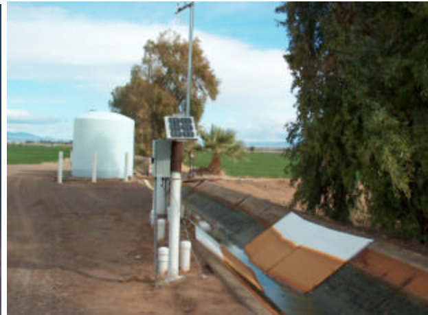
CD100 On-Site w/Solar, Antenna, Steel Box and Bubbler Sensor
